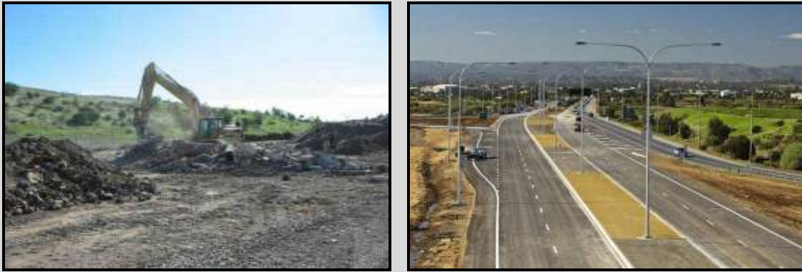
Figure 10.1 (Left) Breaking up recycled concrete (Right) View of Stage 1 of the Port River Expressway
